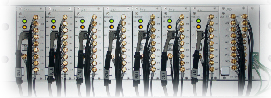
Figure 12: GISmonitor built into a 19-inch rack
